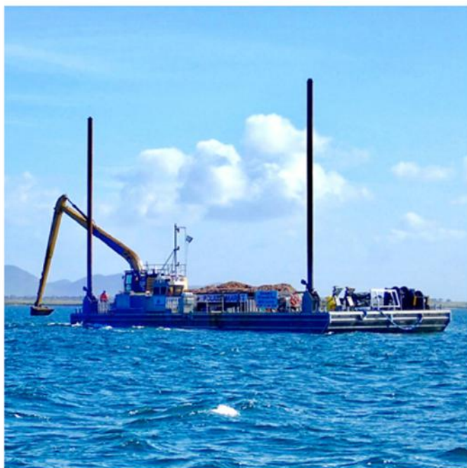
Longreach excavator deploying recycled shell at 9ft Bank in Geelong Arm. Photo: Simon Branigan.
